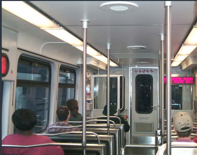
Airflo Light Fixture ICD- 110052
